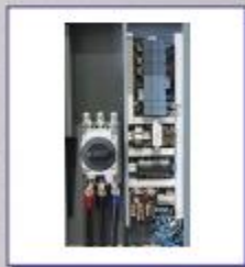
Control panel and Circuit breaker
